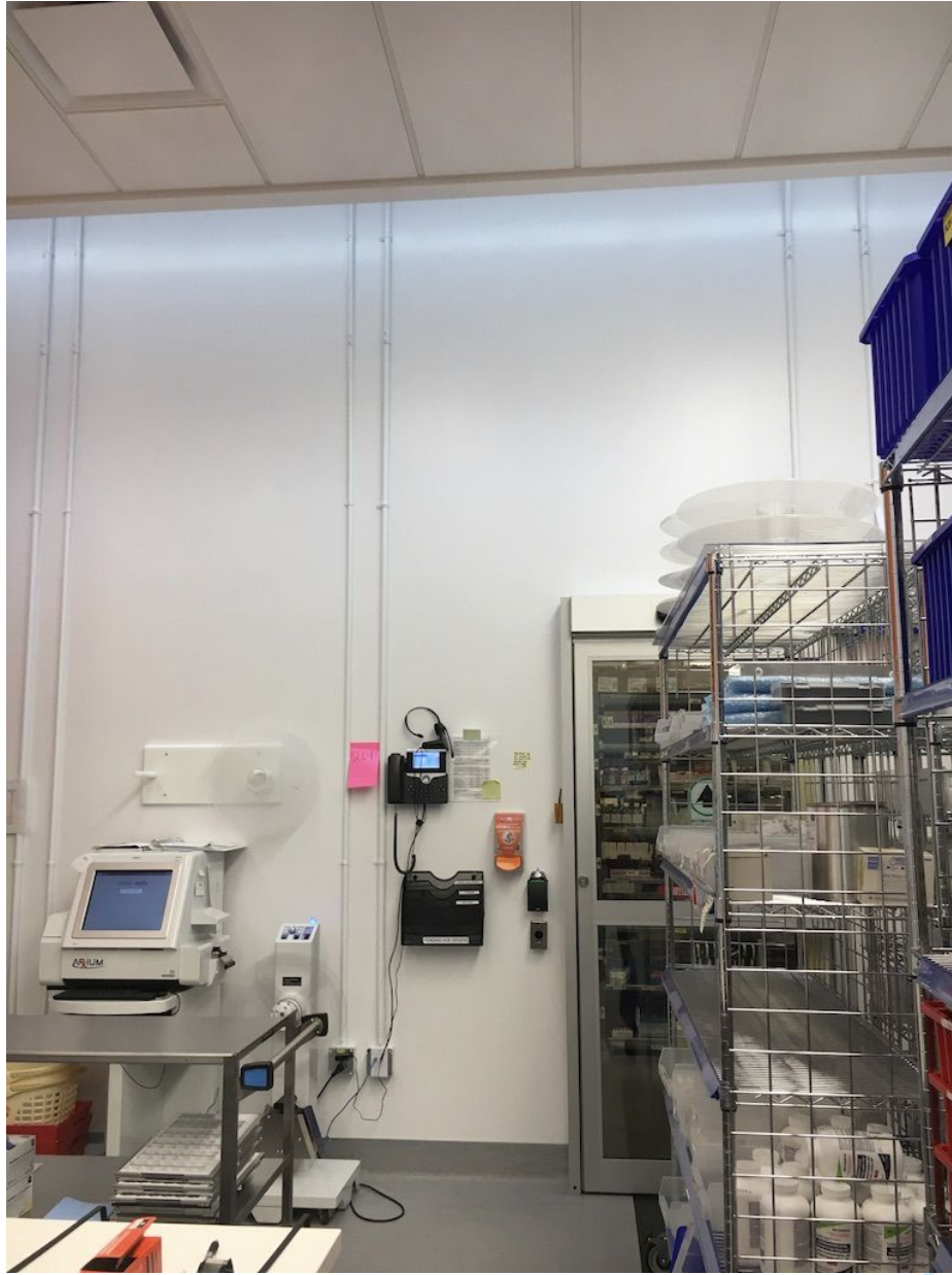
Figure 2. The impression of sky lighting given by circadian lighting installed around a room's perimeter.
