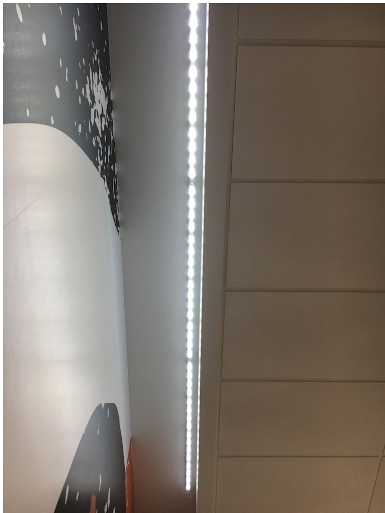
Figure 1. Circadian lighting installed in a recessed crevasse along a perimeter wall.
