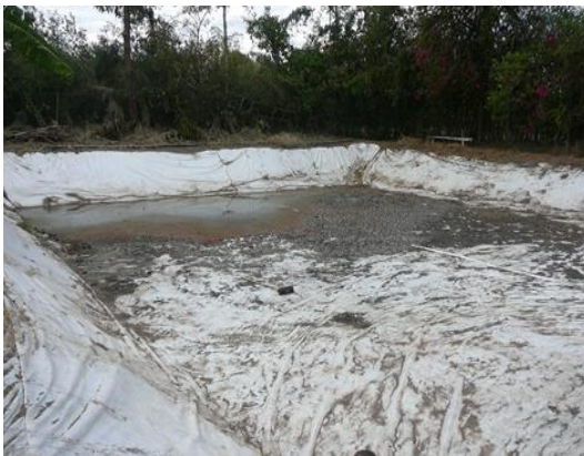
Figure 30: Empty pond with silt due to poor siting and leakage, photo by J.Mang'era
