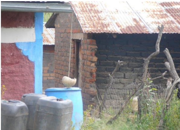
Figure 24: Simple basic roof catchment – Malili, Photo by J. Mang’era
